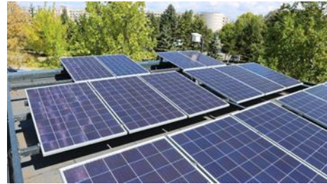
Figure 2. PV system on the roof of the innovative demonstrational pavilion in Sofia with installed capacity 5.04 kWp
